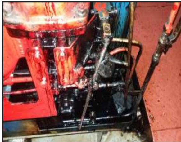
Oil accumulation at few location in the engine room
