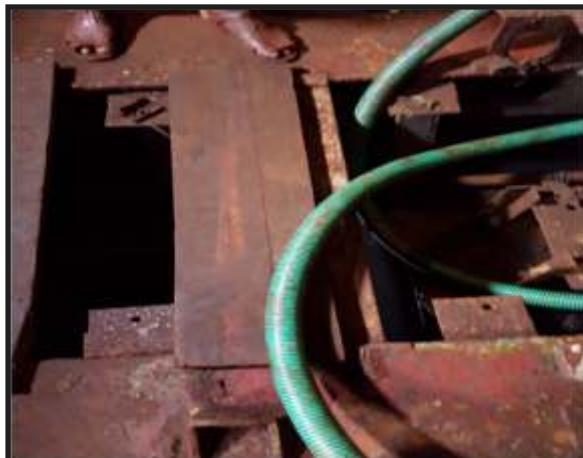
Machinery space without floorplates, and Engineer safety shoes missing
