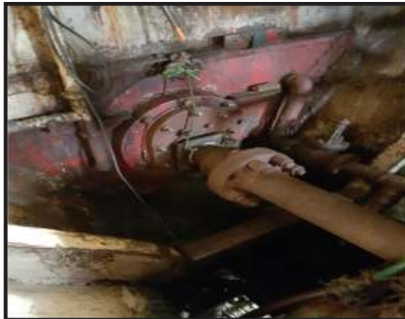
One propeller shaft coupling bolt missing and adjacent areas untidy
