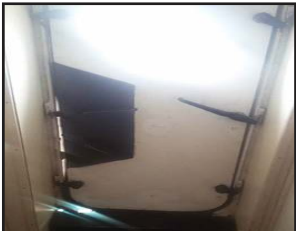
Accommodation Entrance door holed
