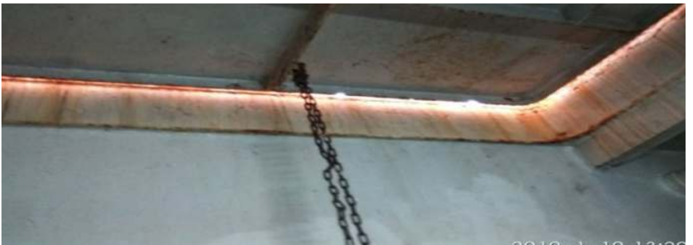
Engine room Skylight door not sealing, packing missing
