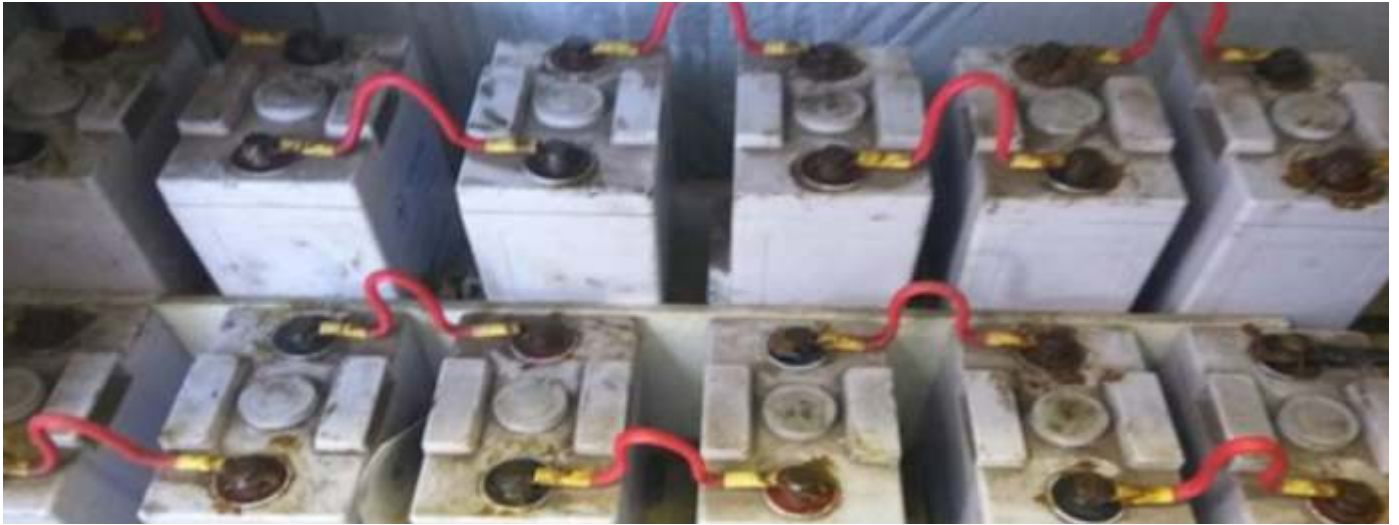
Annual capacity test records of GMDSS batteries are not available
