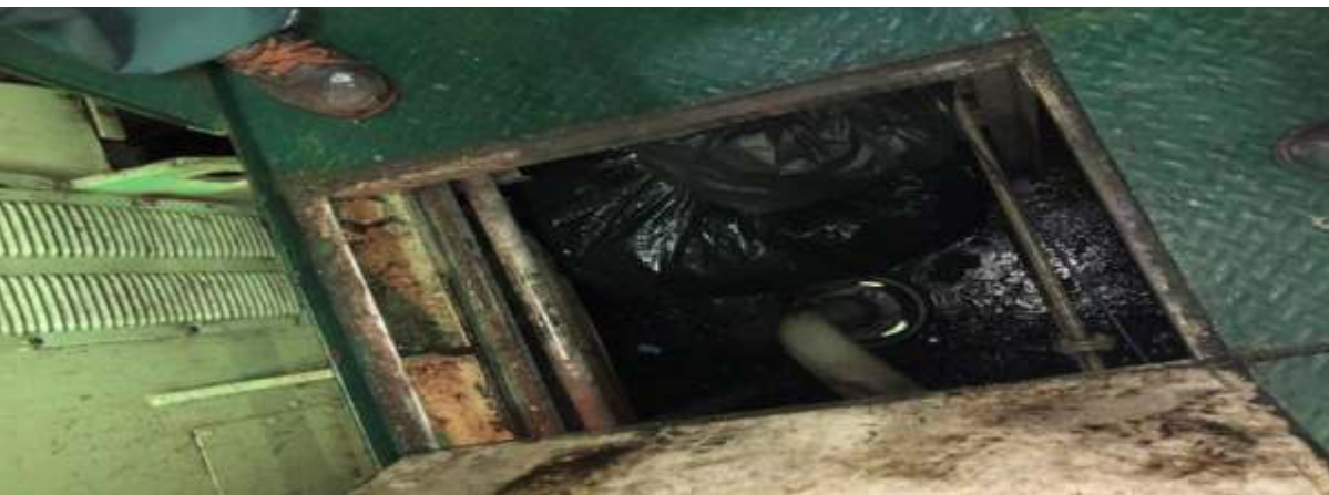
Garbage bags stored under the engine room gratings
