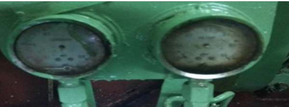
Sludge pump both pressure gauges are defective
