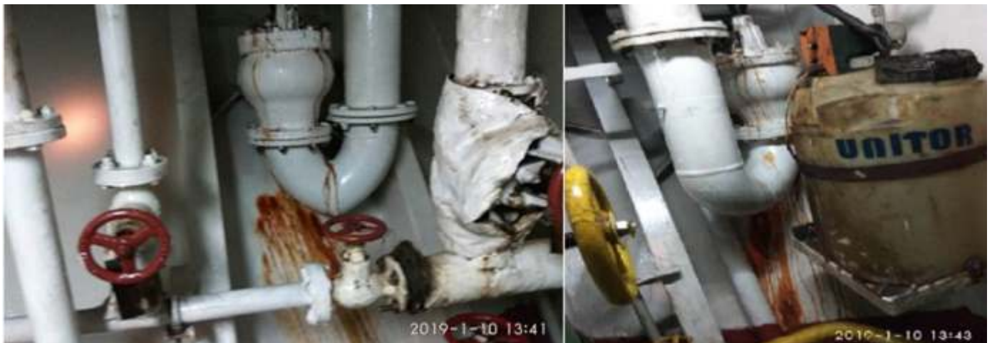
Main sea water pump overboard valve part leaking
